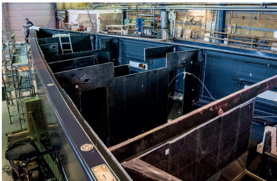
Baltic's construction method allows most systems to be installed at an early stage
